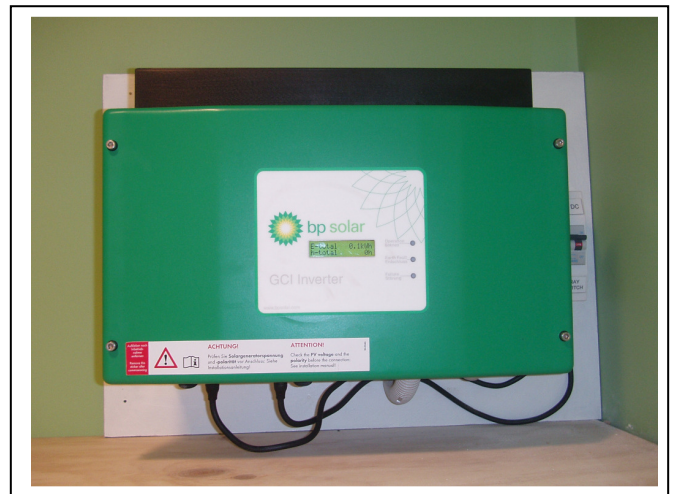
Sunnyboy (BP Solar) 1100E Grid Connect Inverter
